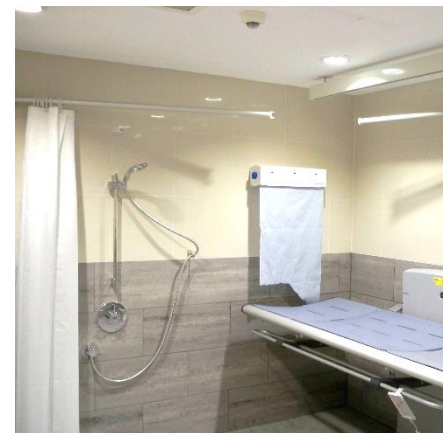
Changing Bench – Air-Side Changing Places Facility
